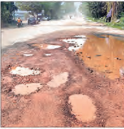
A cracked, broken and dusty stretch of Taratala Road on Tuesday. Picture by Souk Saha
